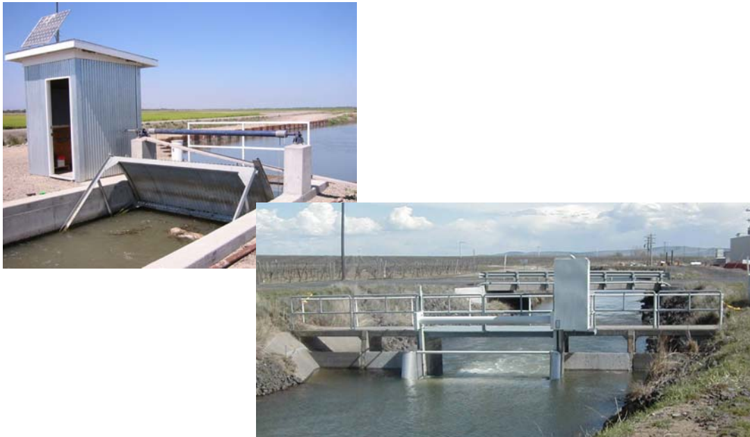
Figure 62. The gate structure and the check structure shown in the photographs have been automated using SCADA. Gate actuators allow for the gates to be raised and lowered from a centralized location.
