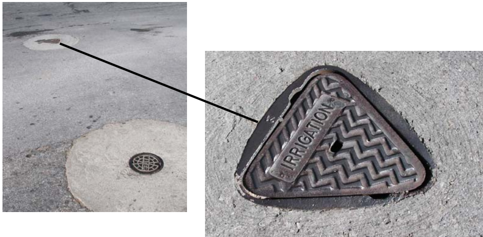
Figure 14 – Secondary System (Irrigation) Valving Access in a Residential Street
