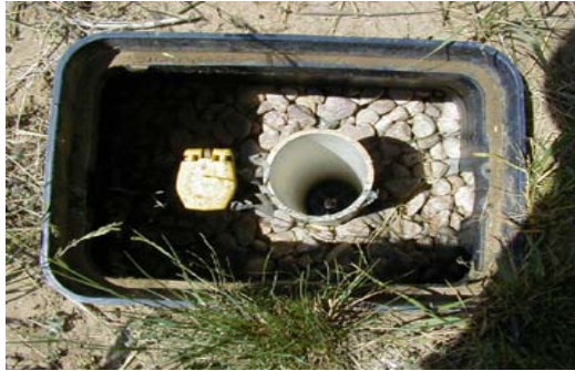
Raw water point-of-connection valve, valve box, and winterization point
