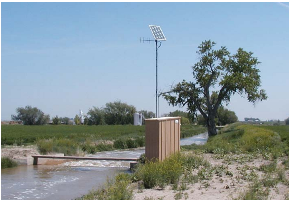
Figure 61. SCADA equipment was installed at this rated section on a canal system in northern Colorado. The existing house for a Stevens recorder was used and a solar panel and remote terminal unit (RTU) was added. Communication is via radio. The equipment is all solar powered.
