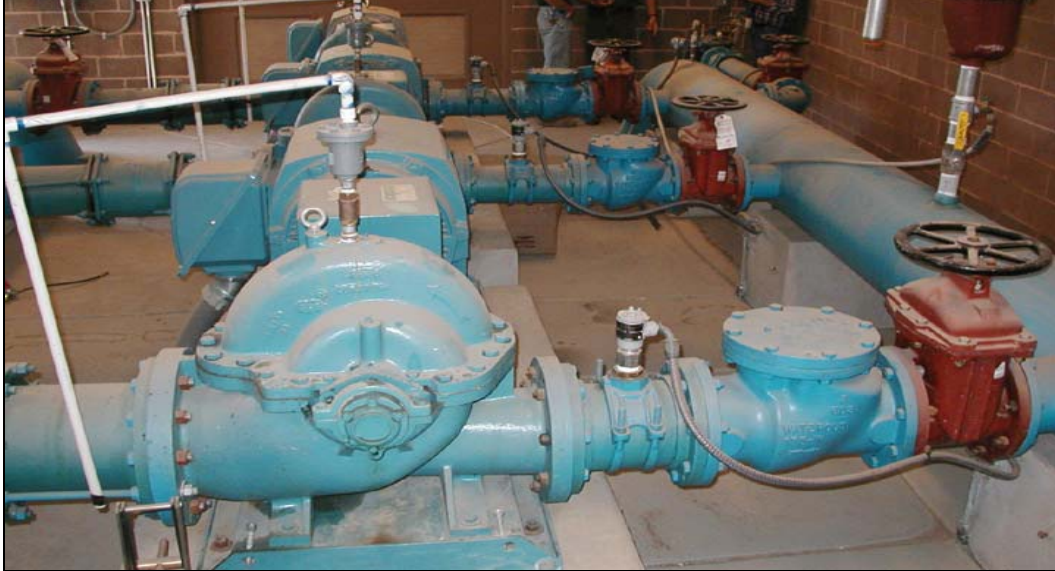
Figure 48 – Pump System Filtering and Pressurizing the City of Highland Secondary System
